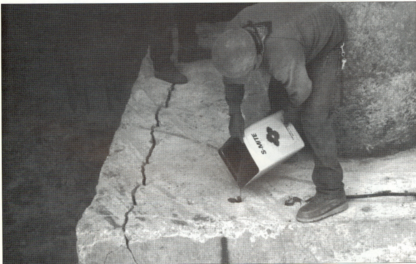
S-Mite is poured into drilled holes along one side of the footing. The crack along the left side of the footing shows the results of the S-Mite after roughly 24 hours of expansion. The crack provides access so a backhoe bucket tooth can pull away the section.
