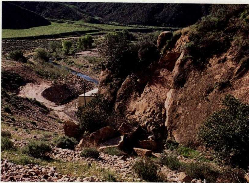
Figure 2 - Wedge-shaped failure that resulted in boulder accumulation along the right dam abutment.
